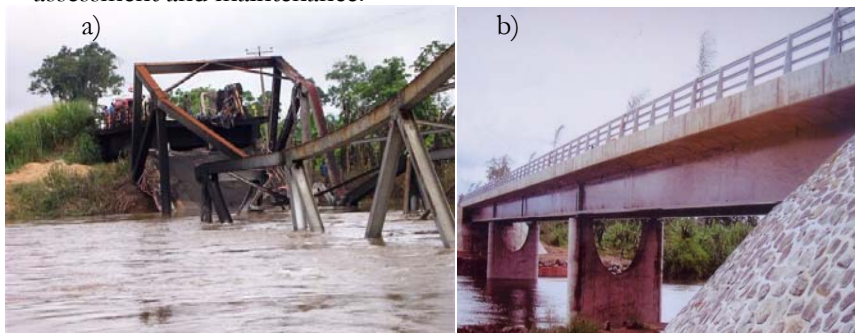
Figure 1: (a) The collapsed former Mungo steel bridge and (b) the reconstructed new one.
